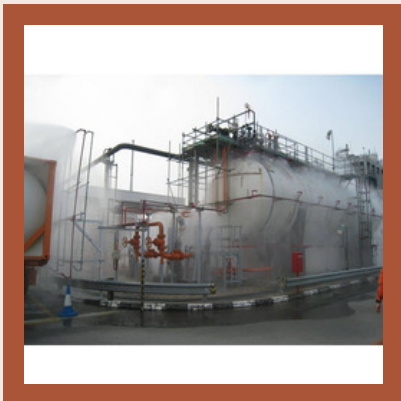
Water Spray System
