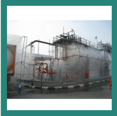
Water Spray System
