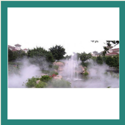
High Pressure Fogging System
