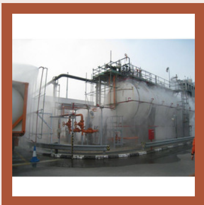
Water Spray System
